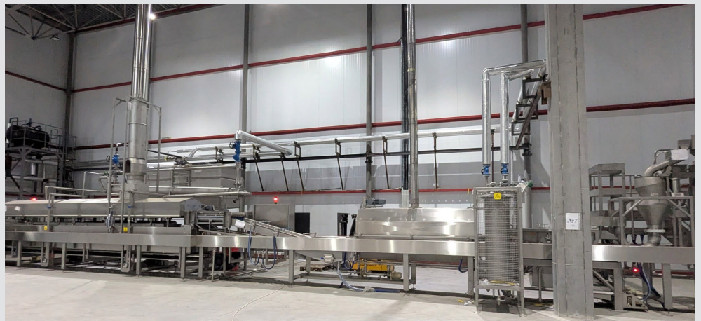
Our PC500 plant installed, November 2025
