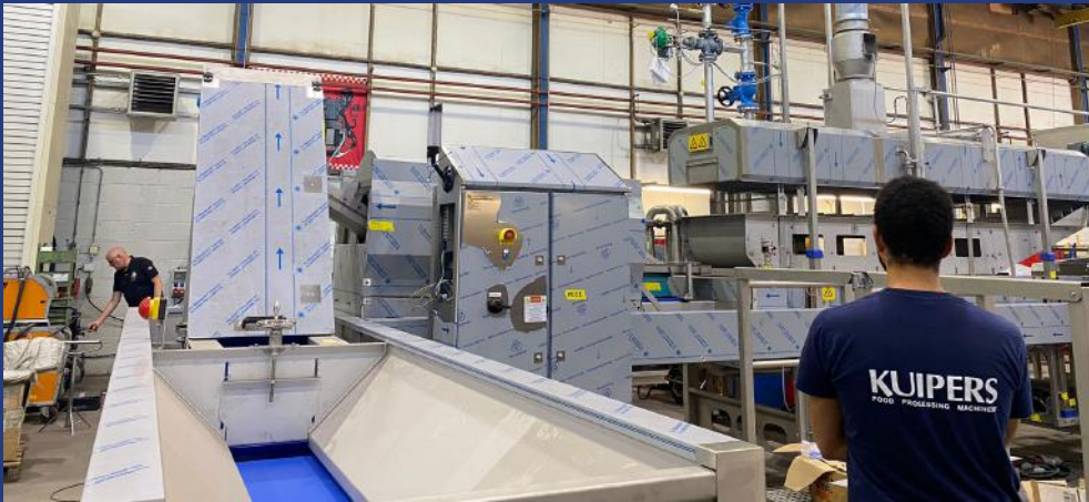
Our PP1000 plant in the Netherlands, June 2023
